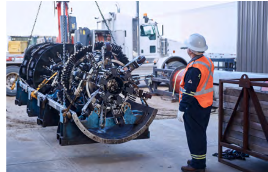
Workers launch an inline inspection (ILI) tool along Enbridge’s Mainline crude oil and liquids pipeline network at Enbridge’s Hardisty Terminal in Hardisty, Alberta. ILI tools move through our pipeline network and use advanced sensors.
