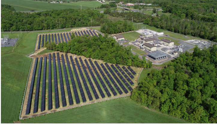
> Solar self-power at the Heidlersburg Compressor Station, PA.
